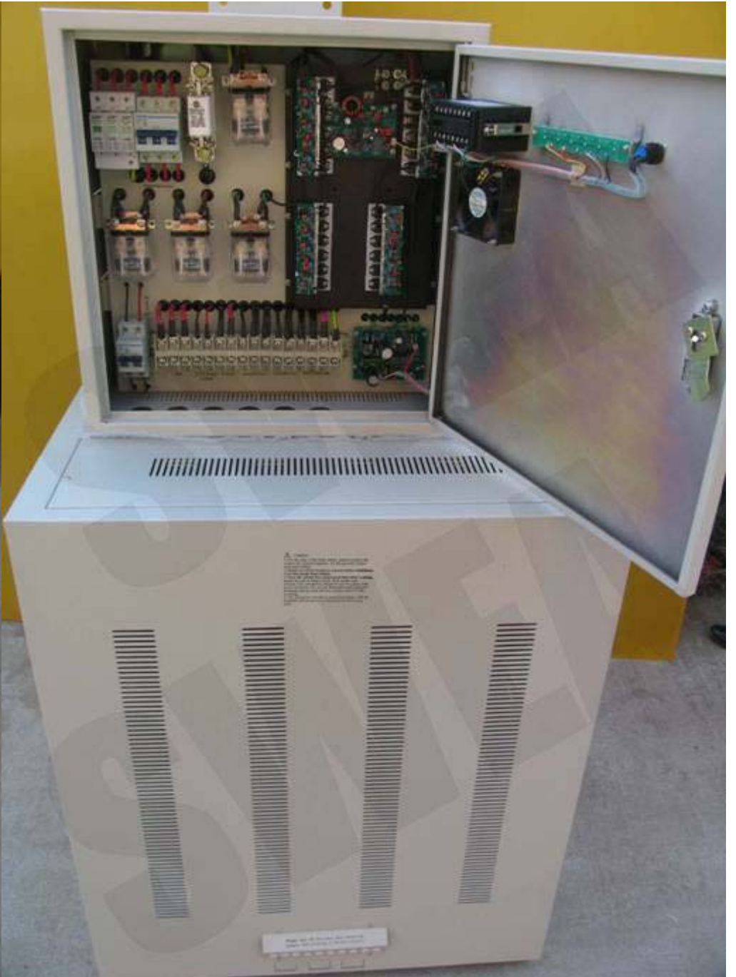
P2. Inside of control system
