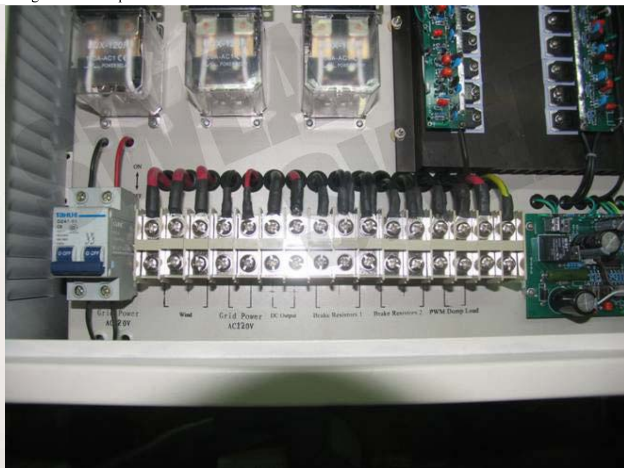
P7. Control Panel Connections
